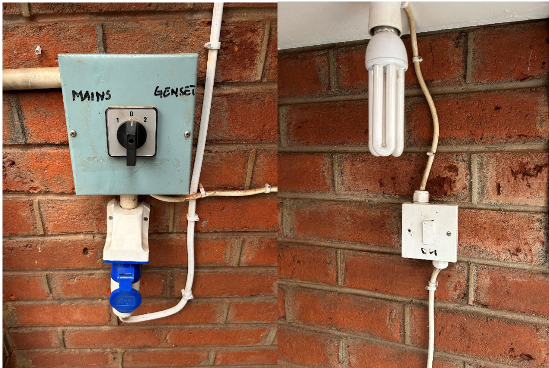
Main Switch outside kitchen Door
